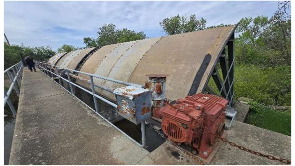
Kelsey Creek Detention Structure
