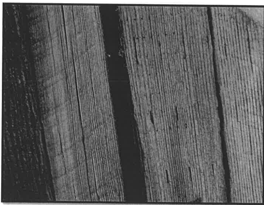
Crevice where bats are found roosting within the existing bridge structure.
