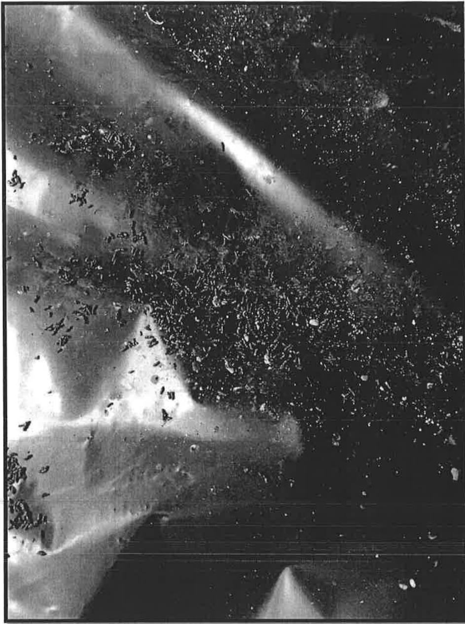
Bat guano discovered under existing bridge.
