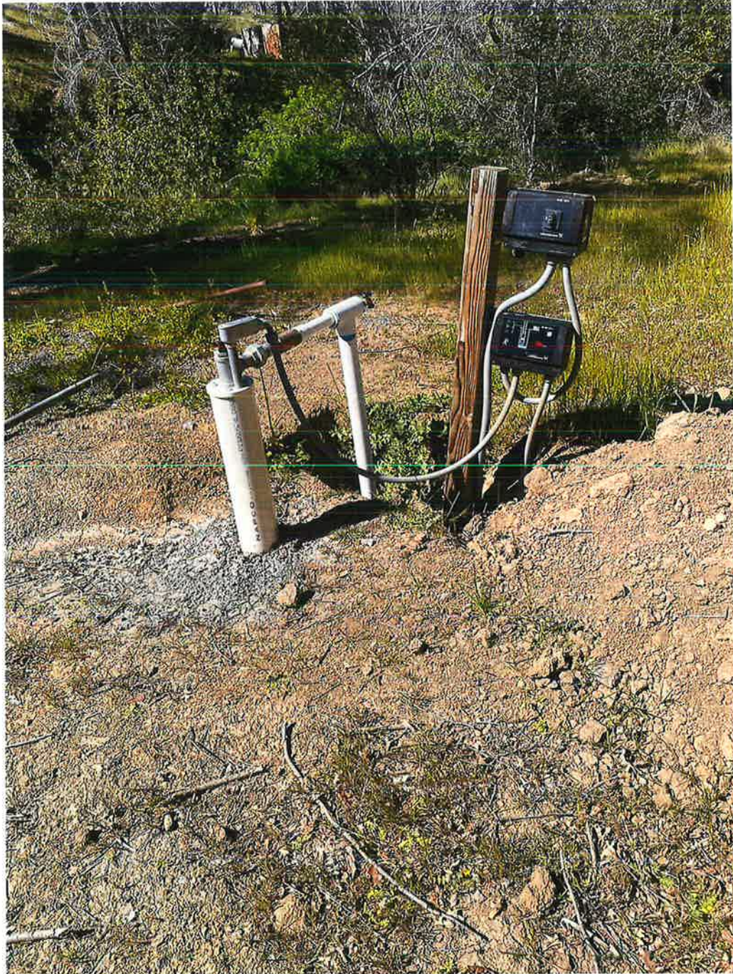
Existing Onsite Groundwater Well
