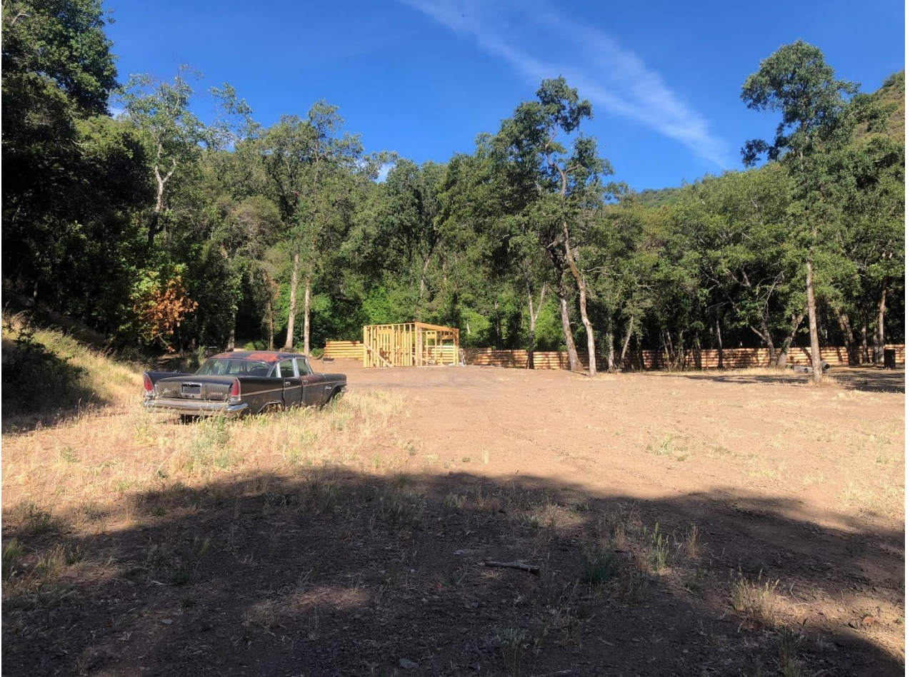
Photo 3. Looking west, this photo shows the cabin in the process of being built. Photo taken on June 17th by Laura Moreno-Baker.
