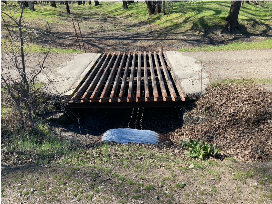
Ephemeral Class II Watercourse Crossing of Comstock Ranch Road – 5' CMP Culvert and 8' Cattle Guard
