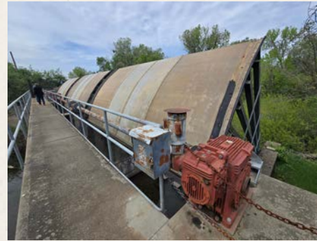
Kelsey Creek Detention Structure
