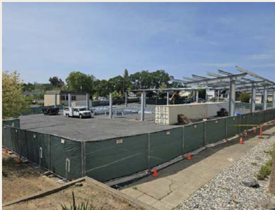
Courthouse Solar Array & EV Charging
