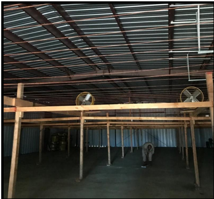
Figure 13. Fans atop drying structure
