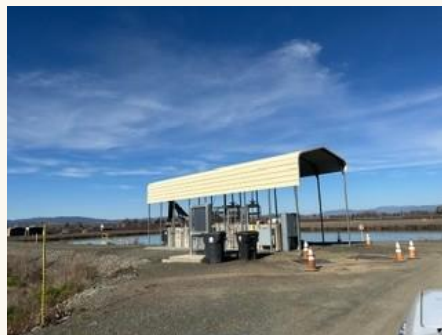
Public utilities like this water treatment plant provide critical services in the Planning Area.
