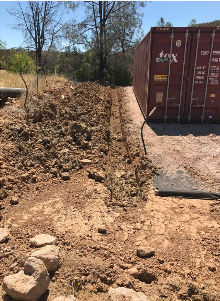
Figures 9-11: Trenching without grading permit
