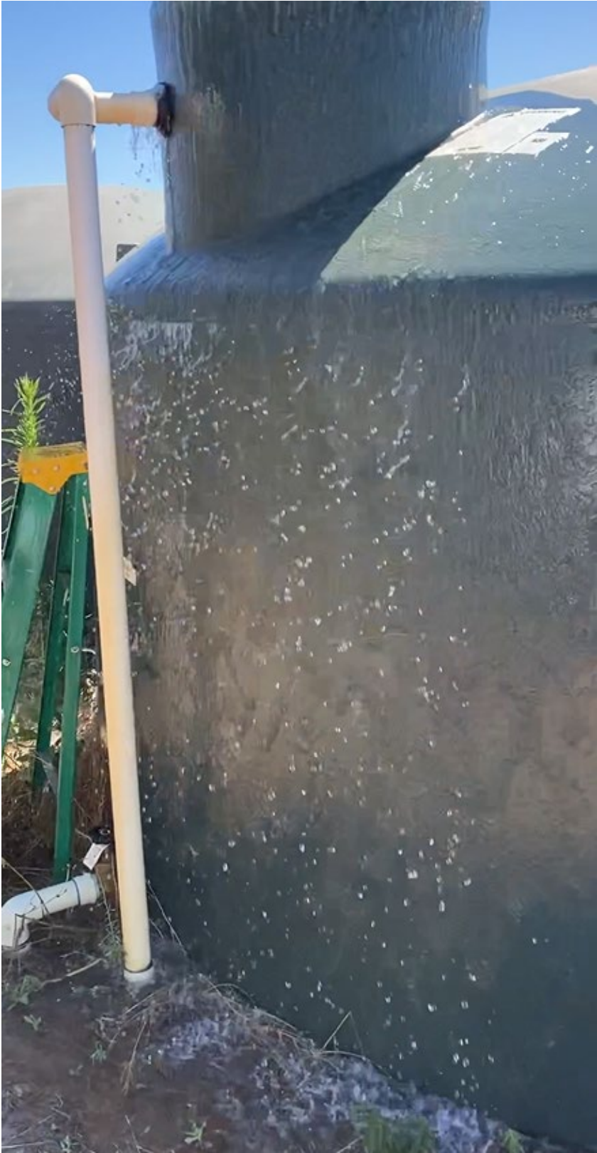
Figure 30: Overflowing water tank
