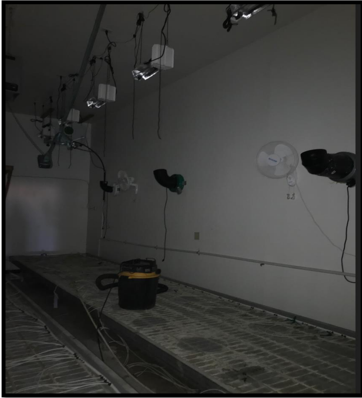
Figure 12. Grow beds, grow lights, oscillating fans, and irrigation systems in second structure
