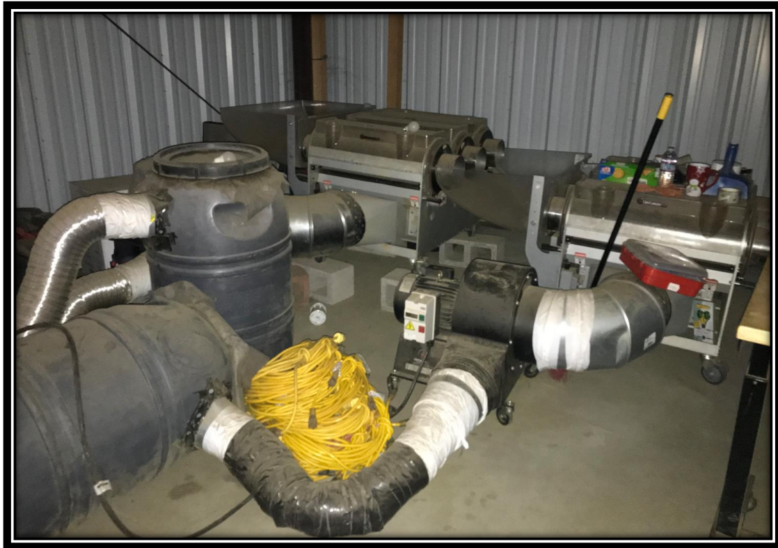
Figure 14. Air circulation system machinery
