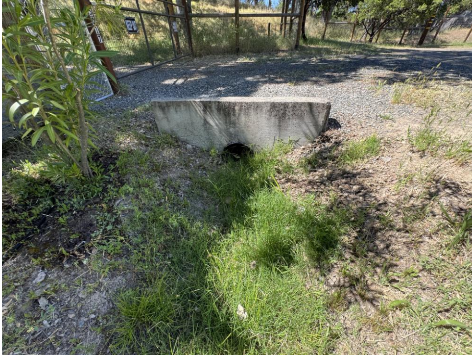
Site Photograph 11 – Looking north at culvert at access point at Terrace Avenue
